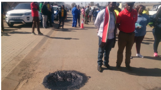
Pothole inside must be properly coated with liner coating
