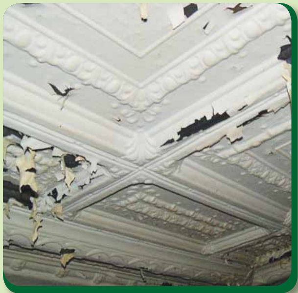
An image of broken asbestos ceiling tiles
