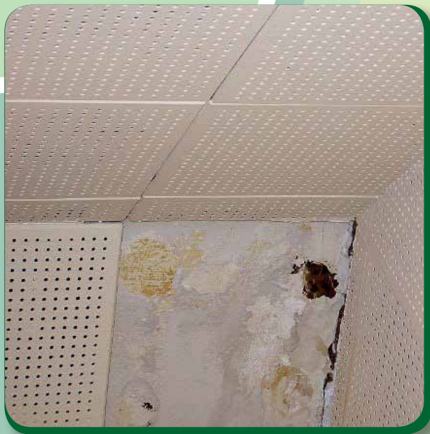
An image of broken asbestos ceiling tiles
