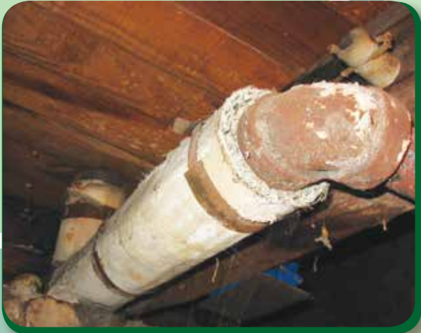
An image of asbestos used in pipe insulation
